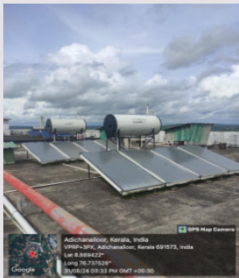
Solar water heater
